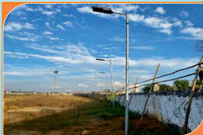
Supply and installation of 65 nos. of Solar Street light at District Sport Association Stadium at East Jaintia Hills District, Meghalaya”
