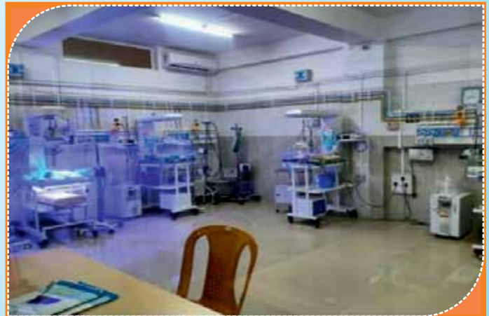
Supply and Installation of Central Oxygen Pipeline at SNCU (Special Newborn Care Unit) at 100-Bedded Maternal & Child Health Hospital Panaliar, Jowai in West Jaintia Hills District, Meghalaya
